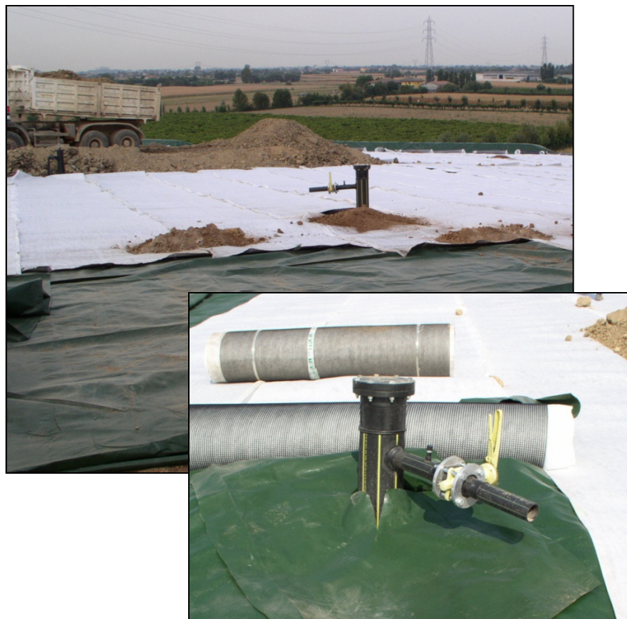
Fig. 6.2 – Disconnection between the vertical shaft and the secondary line
