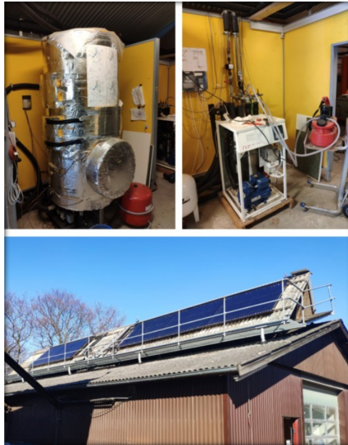
Figure 47: the storage tank (top left), heat pump unit (top right), solar collectors (bottom).
