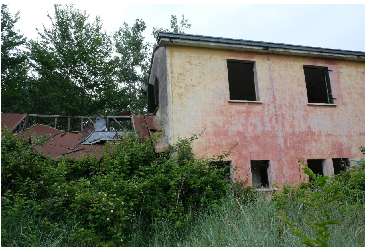
Figure 15: One of the buildings of the abandoned colony, in a state of advanced deterioration.
