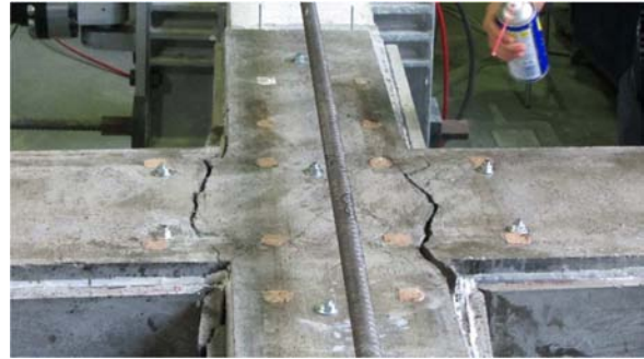
Figure 4.12 – Bending failure in the beam
