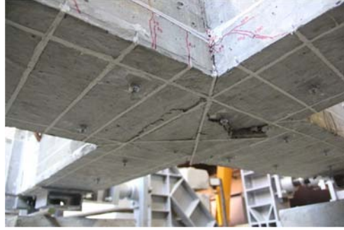
Figure 4.22 – Crack on the bottom surface, JPB joint
