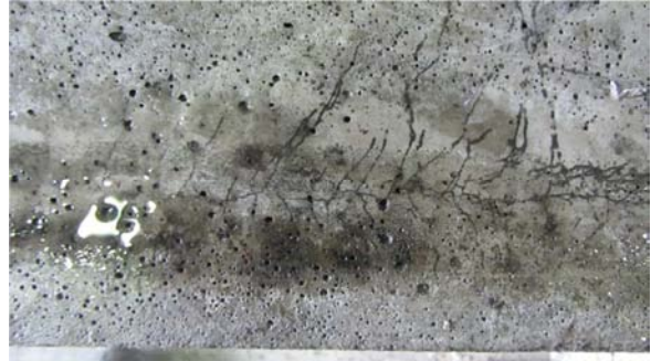
Figure 4.9 – Micro-crack on the SHCC panel along longitudinal carbon laminate
