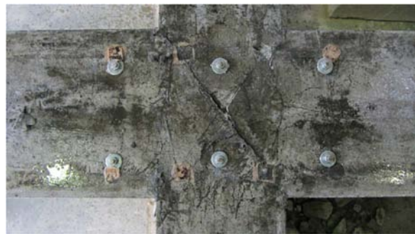
Figure 4.7 – Diagonal cracks in the joint region
