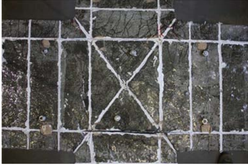
Figure 4.21 – Crack on the top surface, JPB joint
