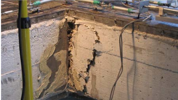
Figure 4.8 - Detachment of the old concrete cover
