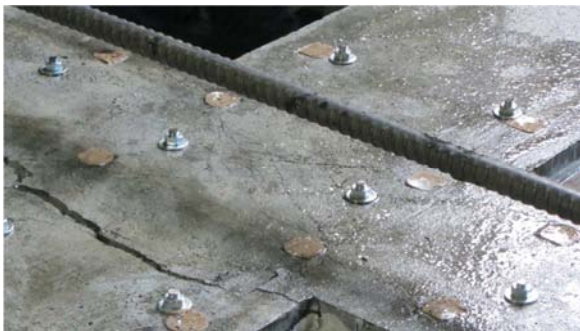
Figure 4.13 – Bending failure in the beam and several micro-cracks in the joint area
