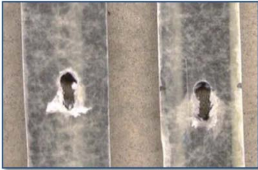
Figure 2.10 - FRP strips failures in MF-FRP system [14]
