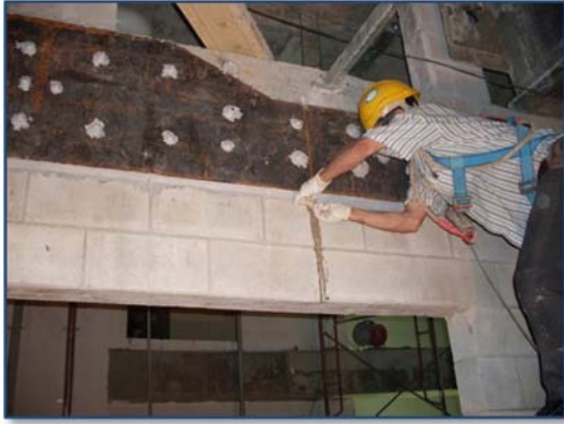
Figure 2.1 – External steel plate [7]
