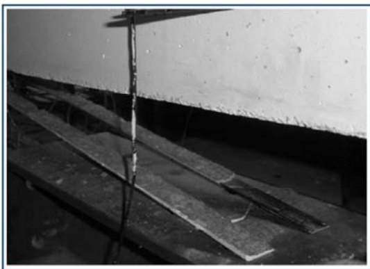
Figure 2.12 – MF-EBR FRP system, bearing failure mode [15]
