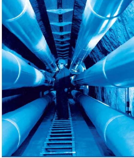
Figure 1.2: Schluchsee Hydro Pump Storage Plant.
