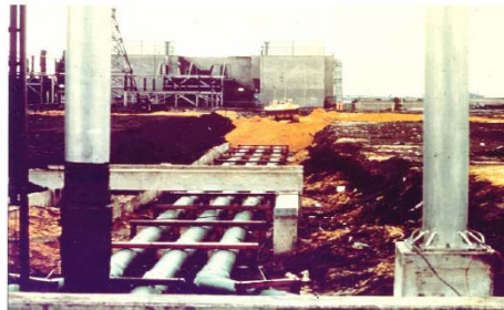
Figure 1.1: 242 kV GIL being installed in the PSEG Hudson generating station. New Jersey. 1972. View looking back from the SF 6 -Air bushings.
