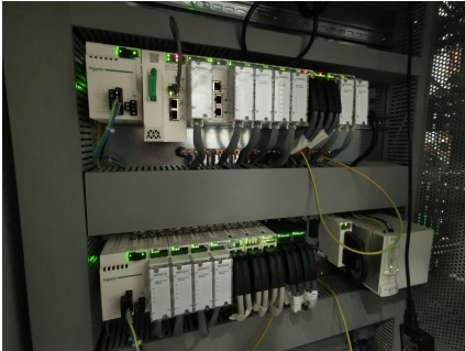
Figure 2.3: Two Schneider M580 PLCs installed in a rack situated in the SPES building.
