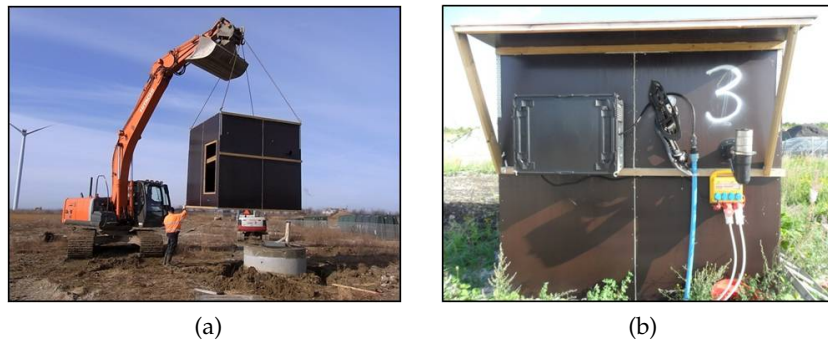
Figure 8: (a): Collection point installation on a leachate well, (b): LFG collection point installed.
