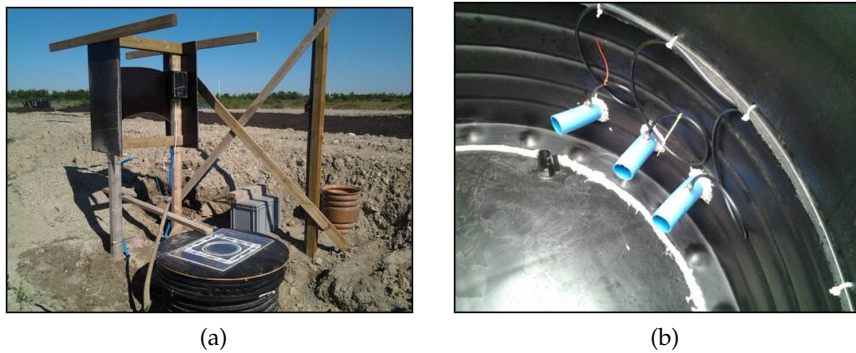
Figure 9: (a): View of the mixing chamber already sealed, (b): LFG inlet pipes inside the mixing chamber.
