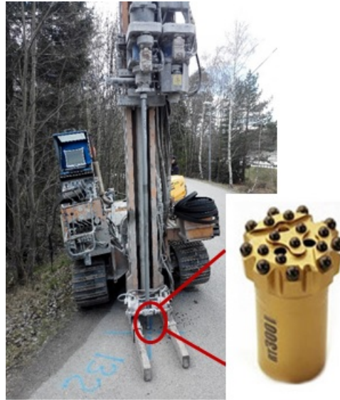
Figure 2.9: execution of a Jb2 sounding in the Dalvägen area (picture taken in April 2016) and the detail of the button bit (indiamart.com).
