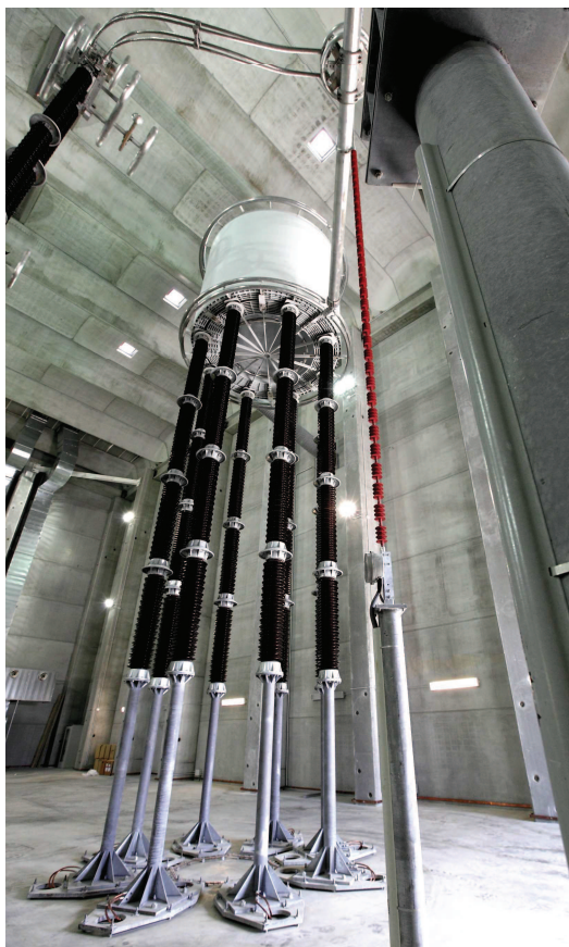
Figura 3.30 – Smoothing reactor isolato in aria, interno la sala valvole
