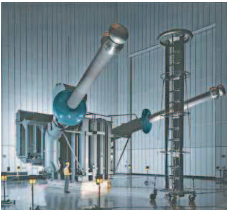
Figura 3.32 – Smoothing reactor da 270 mH, isolato in olio
