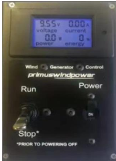
Figure 3-8 digital wind turbine control panel
