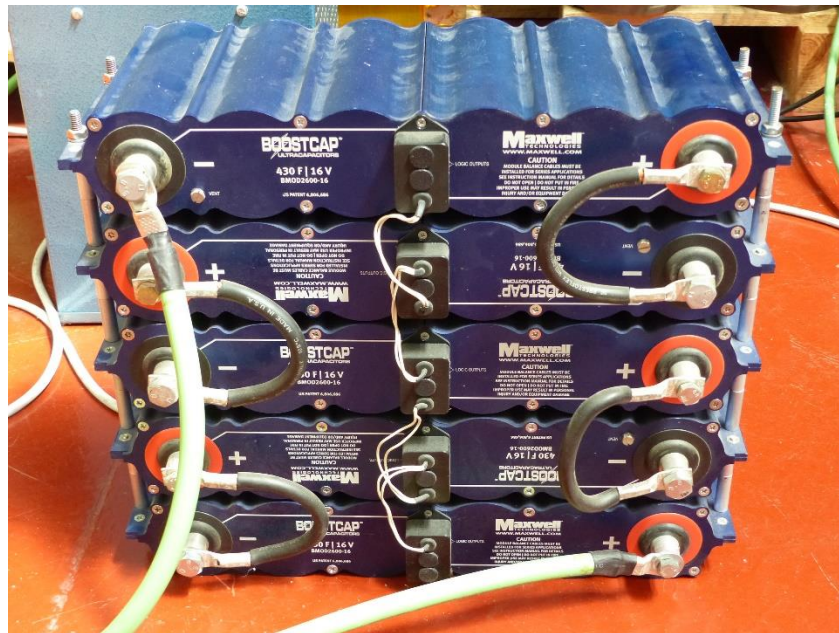
Figure 6.3 – Supercapacitors used in the test bench (5 modules connected in series)
