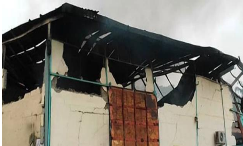
Figure 1.29. Damaged structure of Biopharma's warehouse (cameroon-tribune.cm, 2022)
