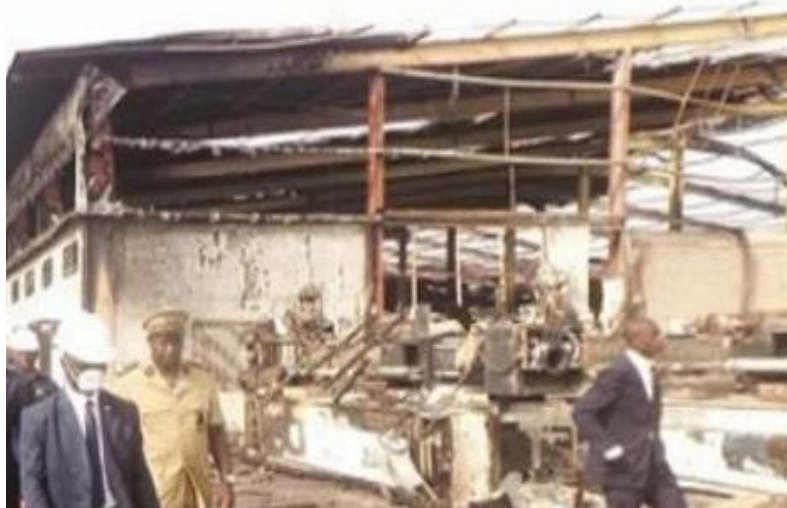
Figure 1.28. Damaged structure of Fermencam warehouses (www.cameroun24.net)
