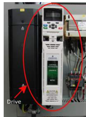
(d) Drive that is in charge of the control of the deviator.
