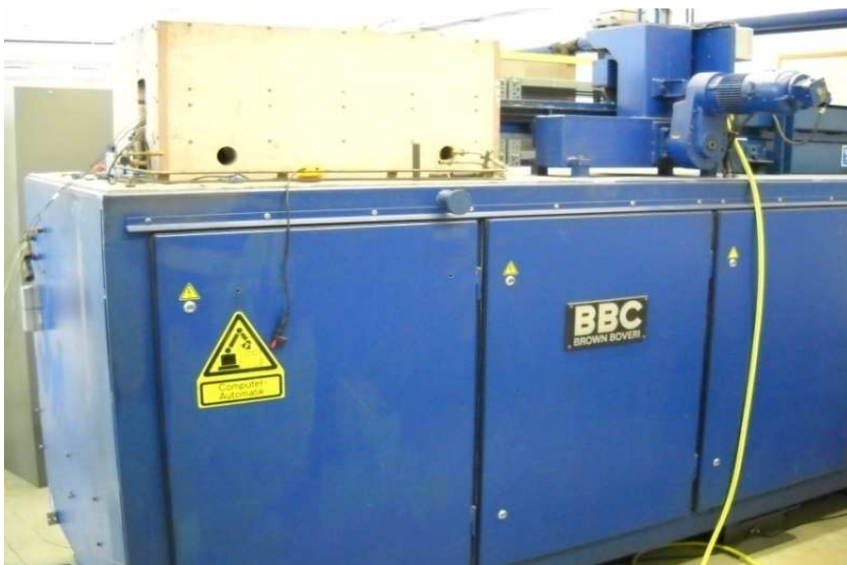
Figure 5.2. Generator used for the experiment BBC Brown Boveri
