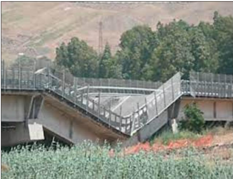
Figure 1.24. Damage and collapse of the Petrulla Viaduct(Anania et al., 2018).
