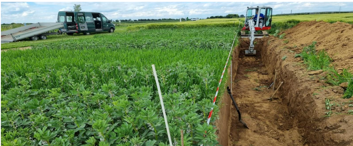
Figure 3: Trench across the experimental field measuring 1.5 m wide and 1 m deep. Source (by Zia Ullah and Arslan) (1 st June 2022) (Location: Campus Klein-Altendorf)
