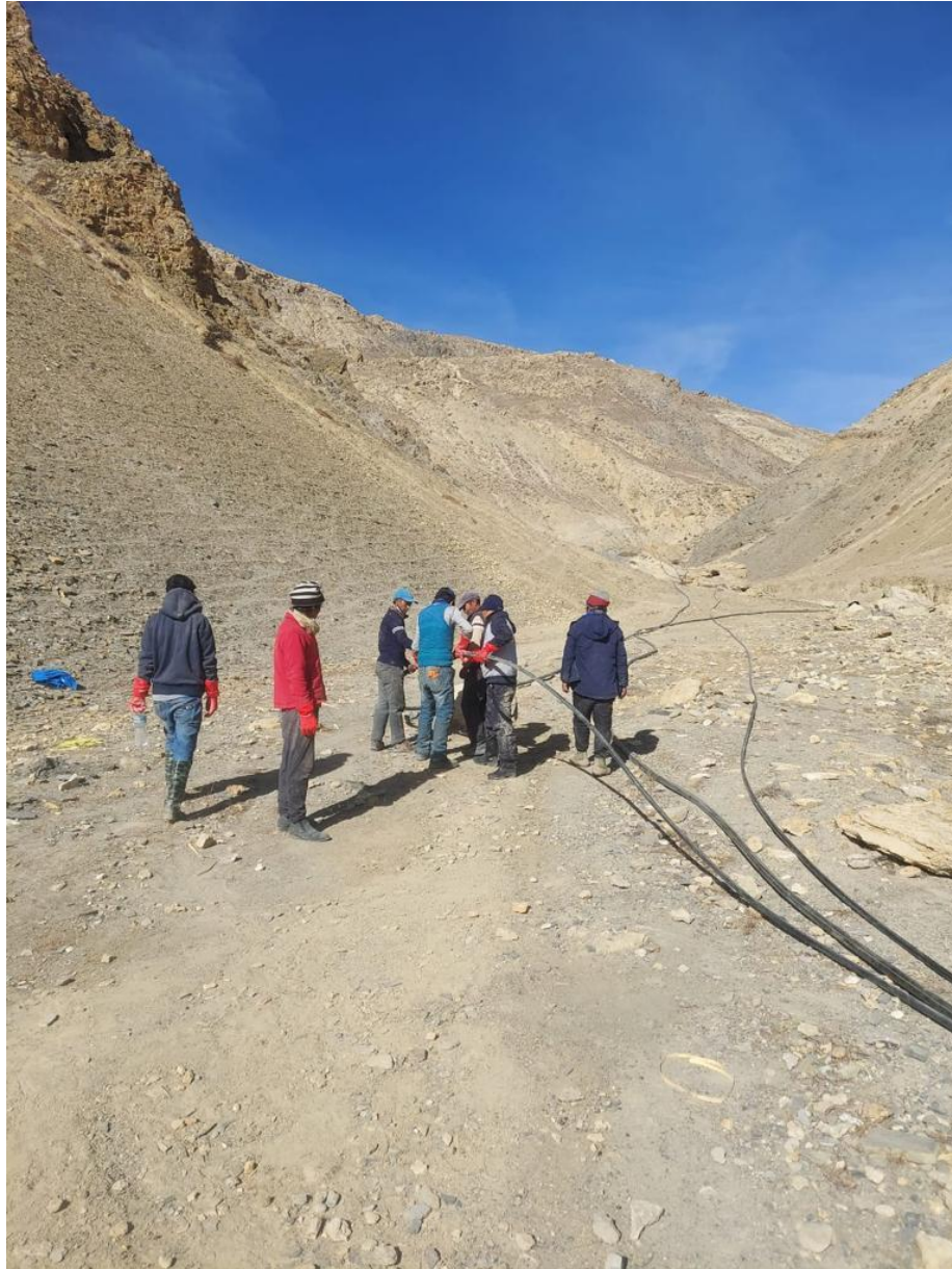
Picture 4. The construction team is bringing the pipes to the construction site of the ice stupa (Videh Foundation, 2022)
