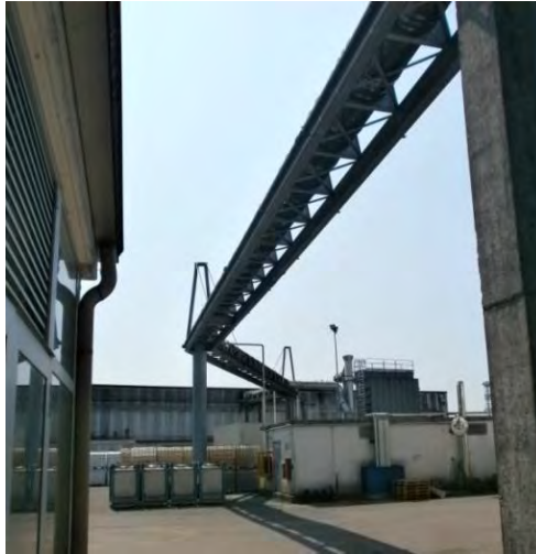
Fig. 3.4.2: Main air pipeline.
