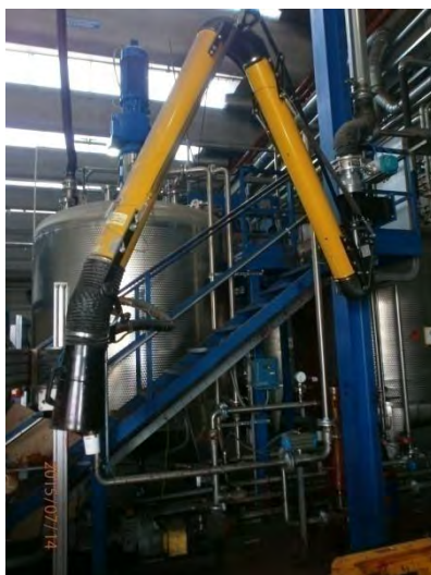
Fig. 3.3.3: Mechanical arm connected to the suction system.
