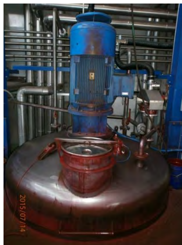
Fig. 3.4.3: Reactor process equipped with aspiration system.
