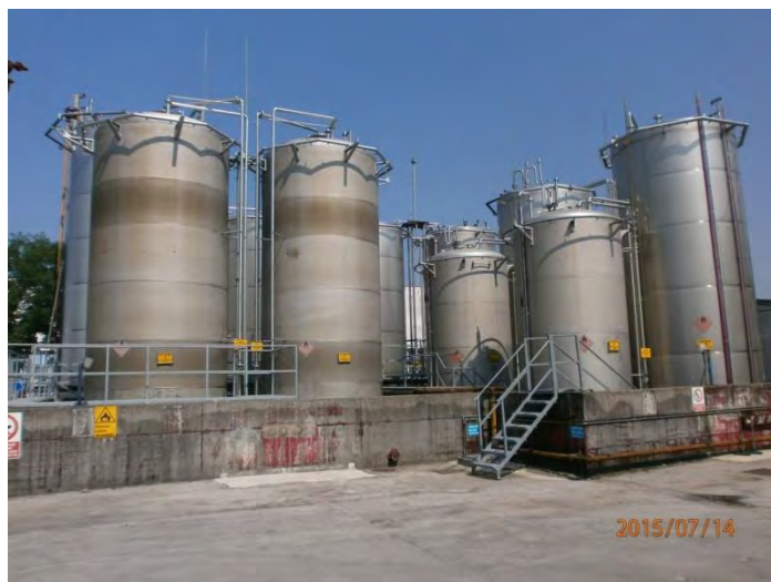
Fig. 3.2.4: Silos for solvents storage.
