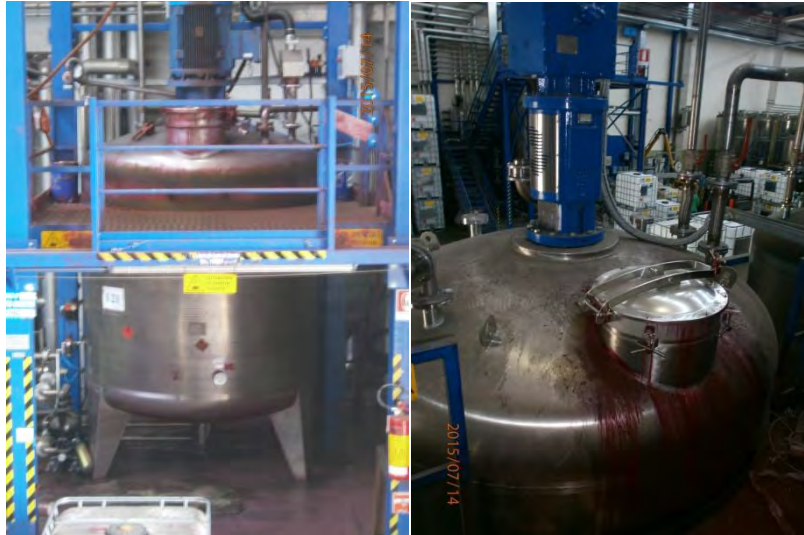
Fig. 3.3.1: a) Mixing station ; b) Detail of the agitator and hatchway .
