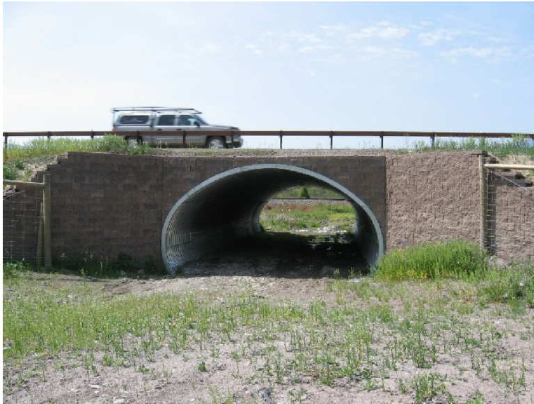
Figure 4.7: Example of large mammal underpass. Image from (Ament).
