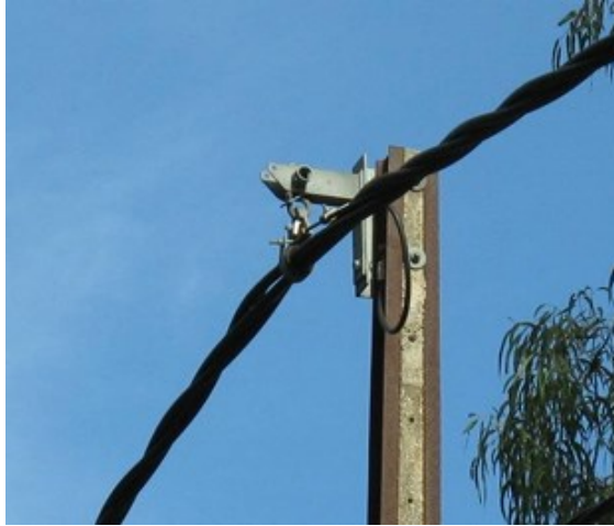
Figure 4.11: Example of insulated power lines. Image from (Australia).
