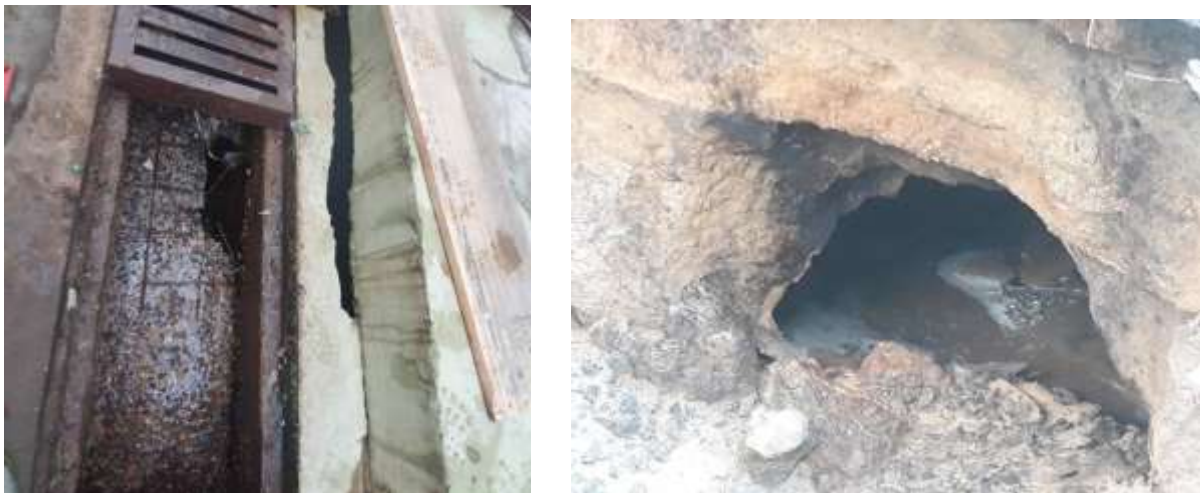
Figure 4.4. Cracks on road pavement (L) – Aging housing water drainage network (R)
