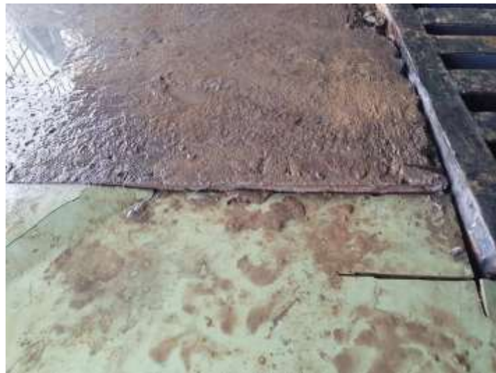
Figure 4.46. Concrete slab fissures at a structure joint (from project data)
