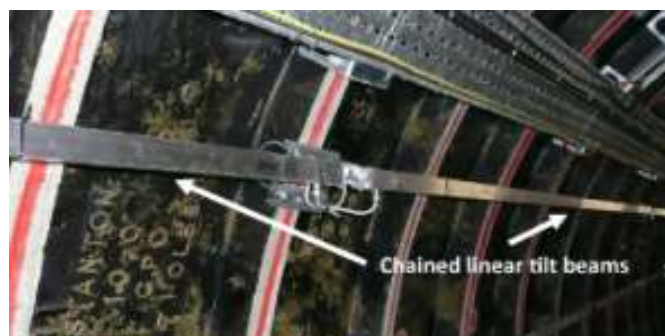
Figure 2.6. Chained linear tilt beams monitoring horizontal movement in a cast-iron bolted lining tunnel (GOESENSE, 2018)
