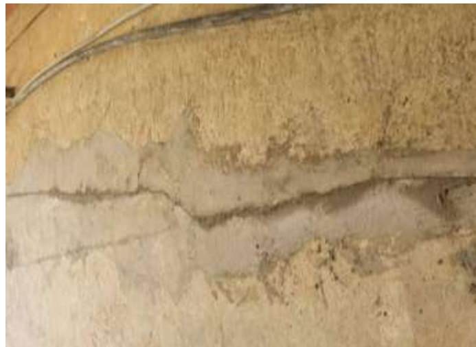
Figure 4.44. Grout getting out the concrete slab (from project data)
