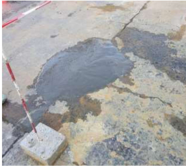
Figure 4.47. Grout rising to the surface through cracks (from project data)
