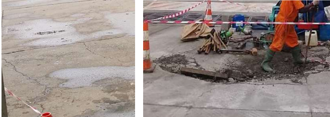
Figure 4.3. Cracks and subsidence sinkholes on road pavement
