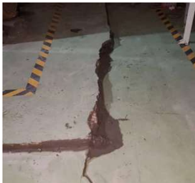
Figure 4.48. Slab breaking post-grouting due to ground heave (from project data)
