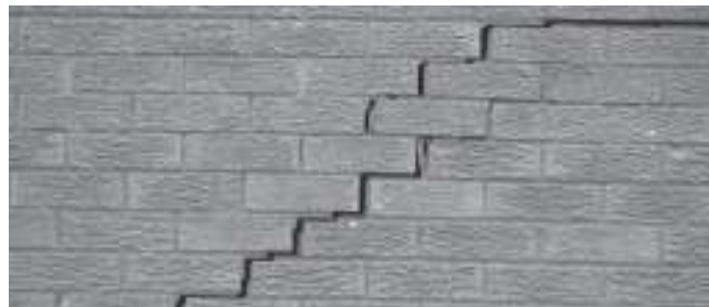
Figure 2.1. Diagonal cracking on structure (Holland, 2012)
