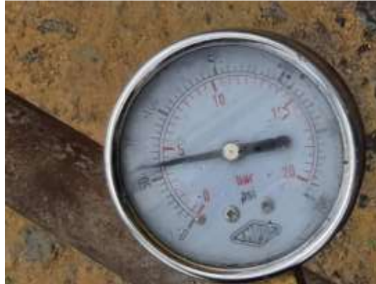
Figure 4.45. Pressure gauges fixed on fittings (from project data)
