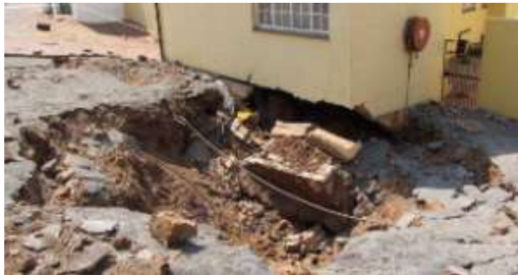
Figure 2.2. Townhouse damaged due to a sinkhole in Gauteng, (Council for Geoscience, 2011)
