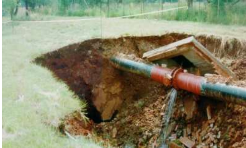
Figure 1.8. Sinkhole due to leakage in Pretoria, South Africa (Council for Geoscience, 2011)
