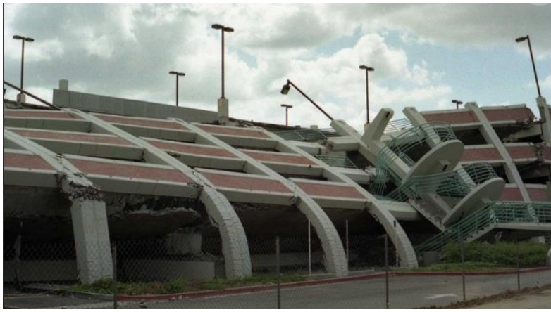
Figure 1. 13. Failure that can occur when the p-delta effect is not taken into account (Mall Parking Structure Collapsed Sideways After 1994 Northridge Earthquake)
