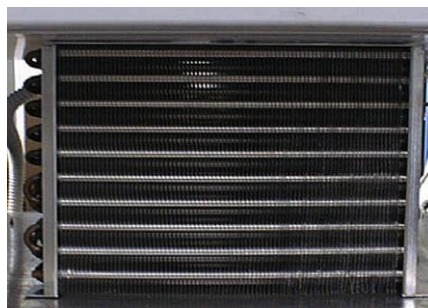
Figura 4.22 – Gas cooler ad aria
