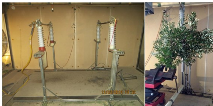
Fig.21 22 kV conductors and vegetation in contact
