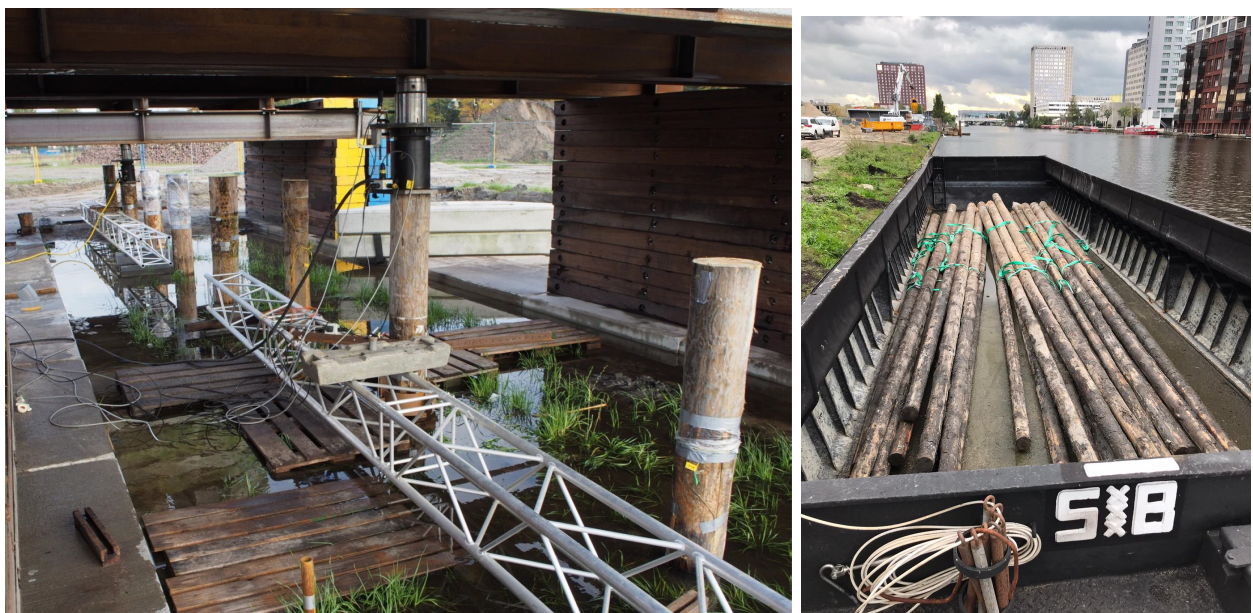
Figure 4.0.1: pre-load in situ of piles driven in Amsterdam, 2019 (left); timber piles extraction and storage in Amsterdam, 2021 (right);
