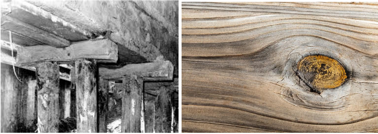
Figure 1.0.1: details of wood piles in Amsterdam (left) and wood knots in timber pile (right)
