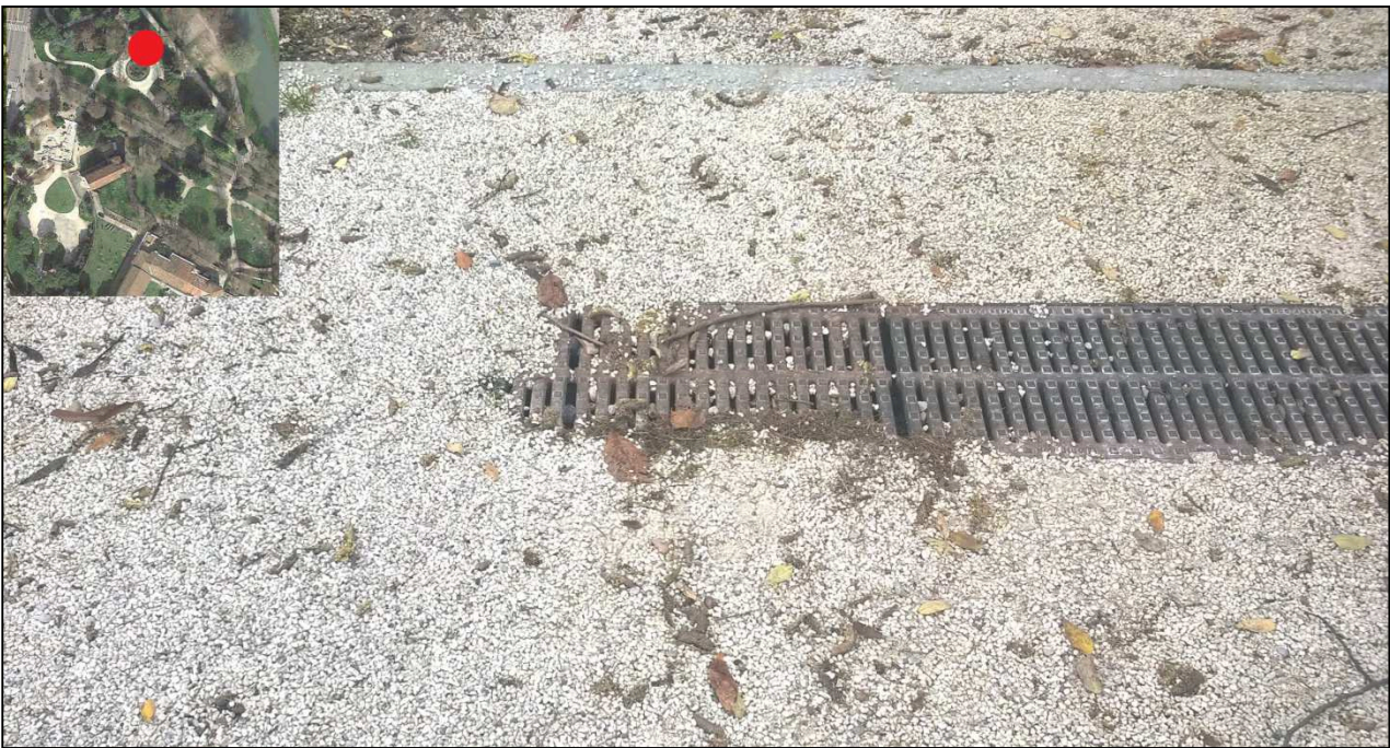
Figure 3.11 Bad disposal of manholes that don't work as hypothesized
