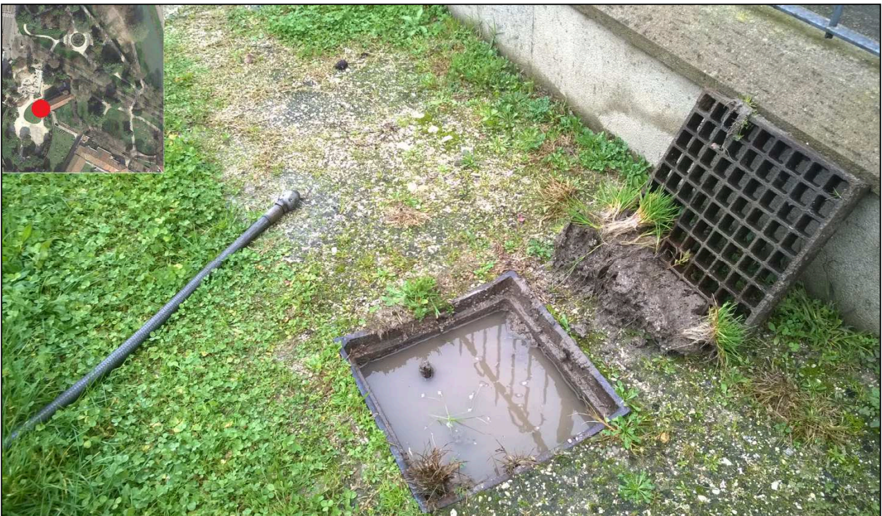
Figure 3.1 Manhole in front of the Chapel, totally clogged by sludge.
