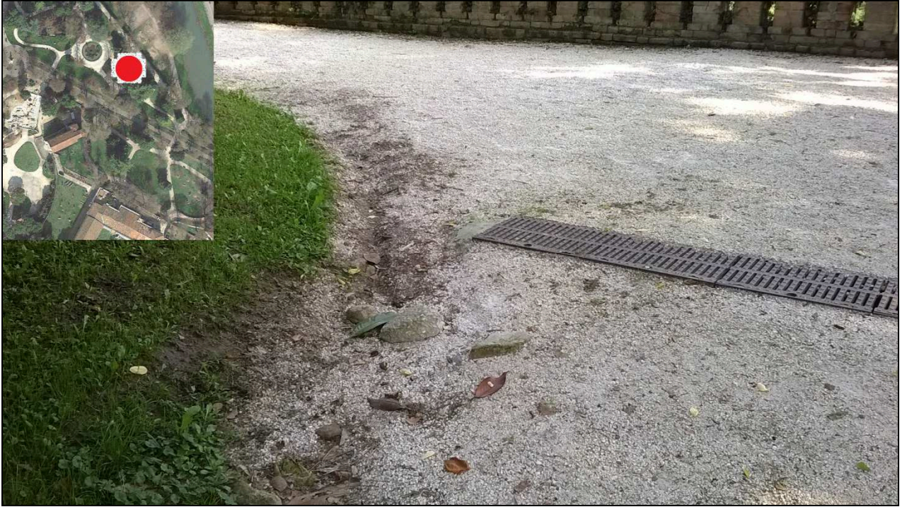
Figure 3.8 Bad disposal of manhole, turned around by rainfall
