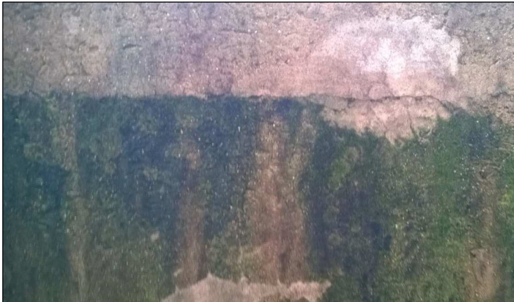
Figure 3.20 Clear level of humidity in the wall around the chapel
