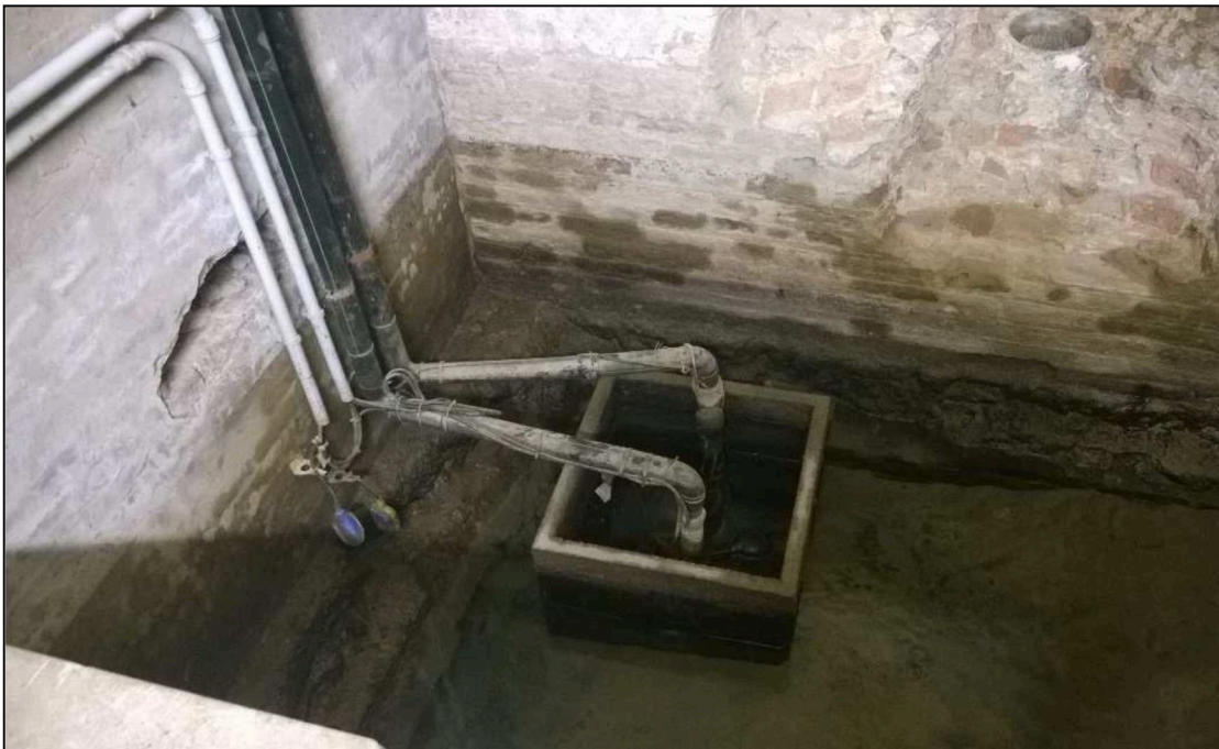
Figure 2.5 Pump station installed inside the Cenobio.
