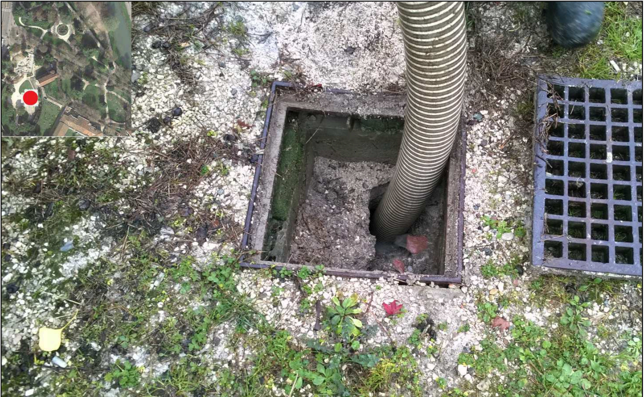
Figure 3.2 Manhole in the Scrovegni totally clogged by sludge
