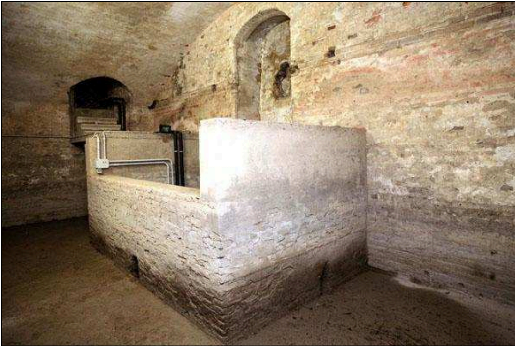
Figure 2.5 Tank containing pumps installed in the cenobio.
