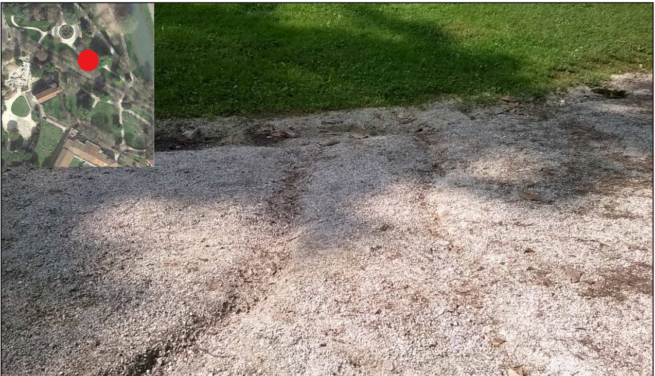
Figure 3.9 Rills in the soil due to a huge quantity of water.
