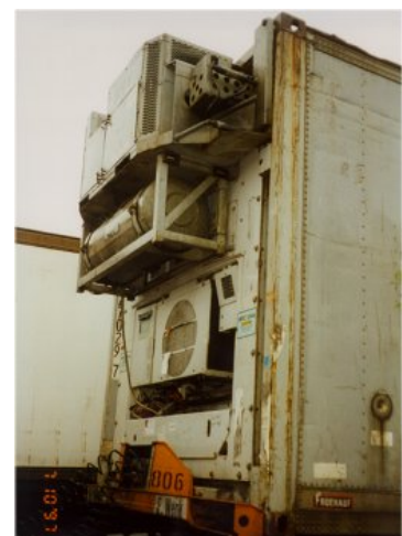
Figure 21: integral unit operated by a generator Source: tis-gdv.de
