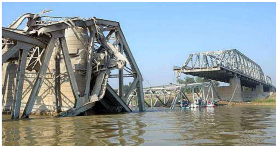
Figure 1.12. Collapse of the Al-Sarafiya Bridge due to blast (NBC News, 2007).
