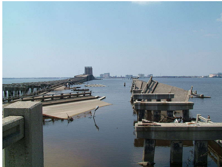
Figure 1.6. Bridge decks knocked off pile caps during hurricane to Biloxi Bay Bridge (Robertson et al., 2007).
