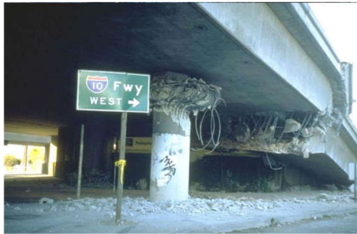
Figure 1.3. Insufficient confinement of columns (Northridge, California 1994).
