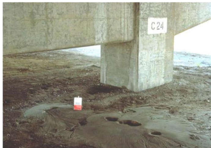
Figure 1.4. Liquefaction (West Grand Viaduct, Loma Prieta, 1989).
