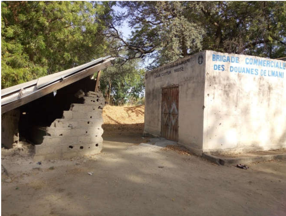
Figure 3.3. Destruction of buildings, impact of bullets on walls and abandonment of administrations (Source: DOA,2018).
