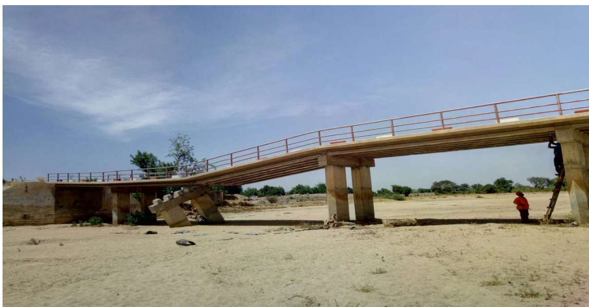
Figure 3.5. Damaged part of the bridge (Source: DOA,2018).
