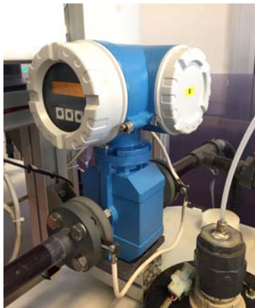
(a) Flow meter
