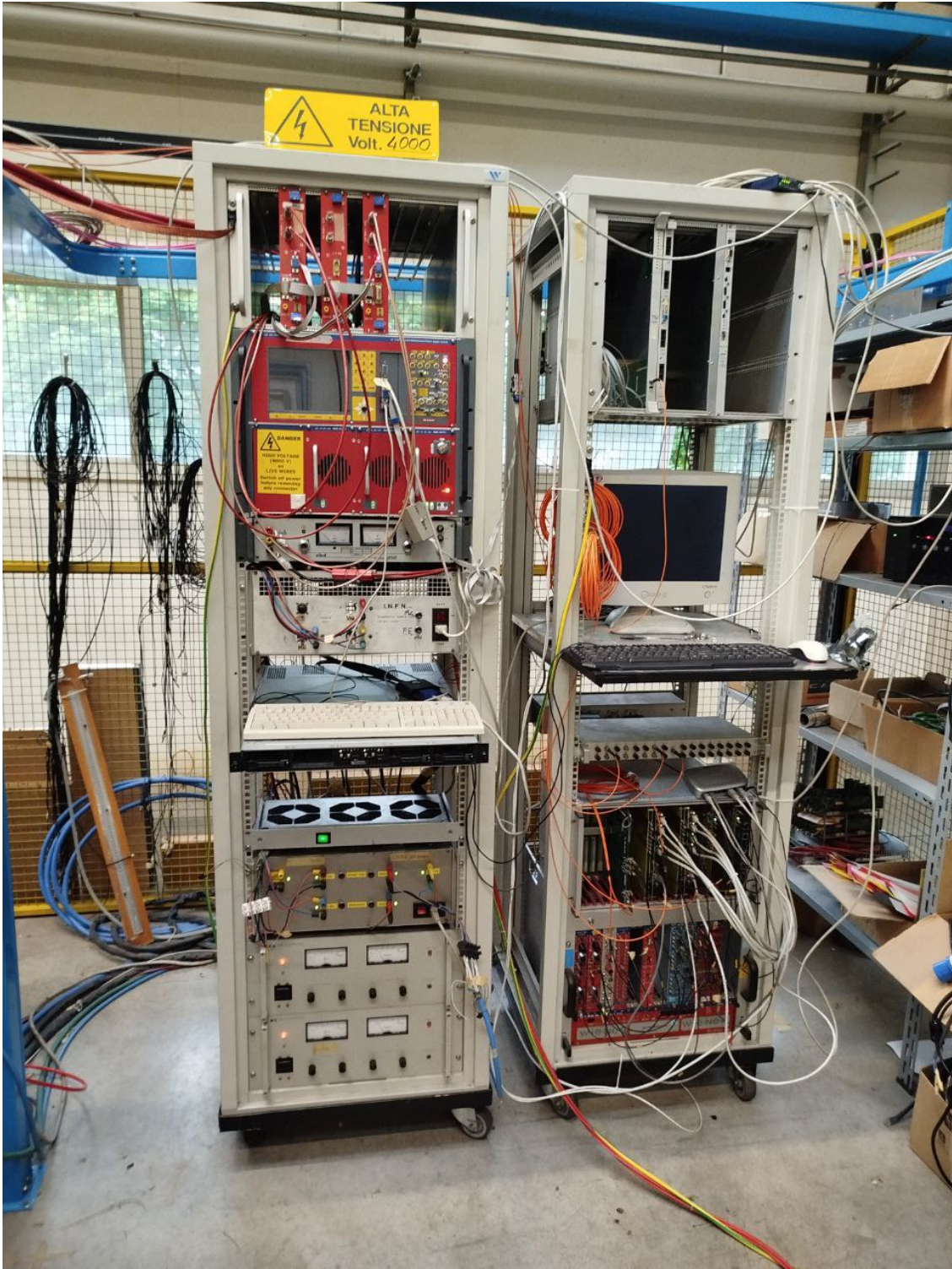
Figure 3.3: high-voltage power supply and data acquisition equipment.
