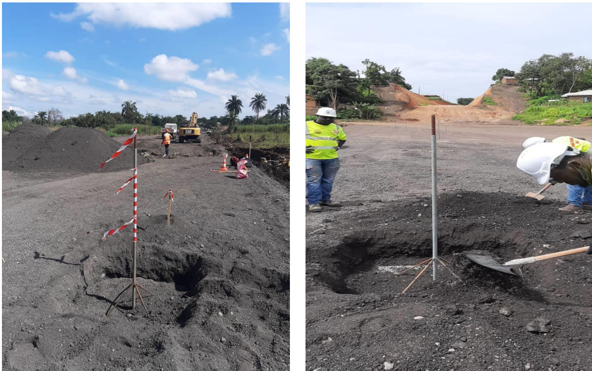
Figure 3.9: Field instrumentation with settlement plates on the pozzolana layer
