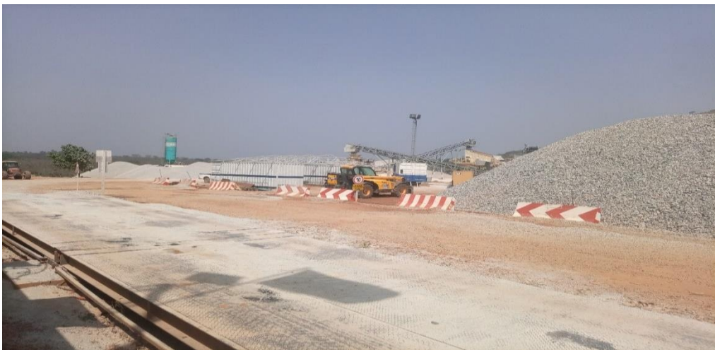
Figure 3.4: Quarry from the section 2 (Foumbot - Bamendjing - Galim) of the project PK 21+250 m
