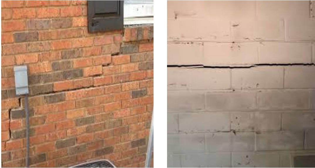
Figure 1-12: Horizontal cracks on masonry wall
