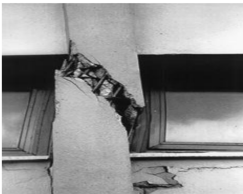
Figure 1-20: Shear failure on column
