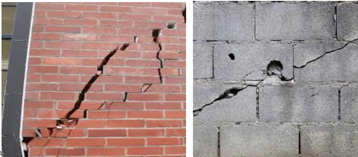
Figure 1-14: Diagonal cracks due to compressional forces on wall
