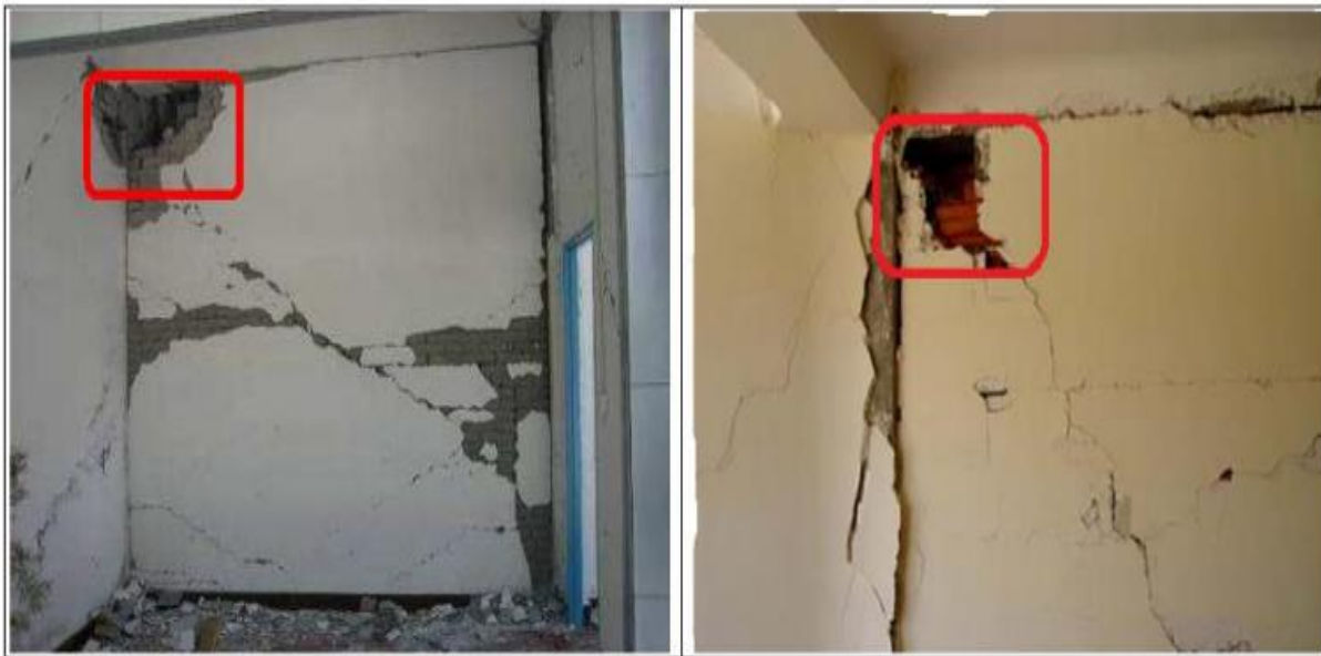
Figure 1-15: Corner-crushing occurring on masonry wall.
