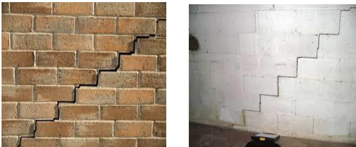
Figure 1-13: Step cracking along mortar joint on masonry wall.
