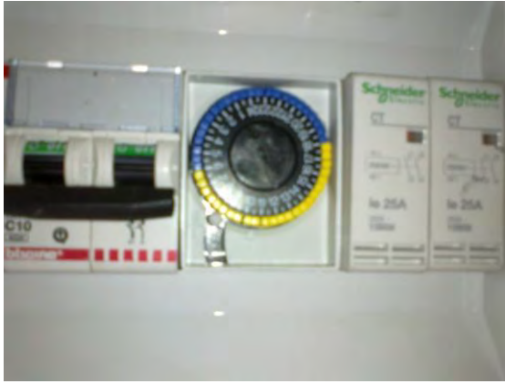
Figure 23. Automatic switcher installed in the greenhouse
