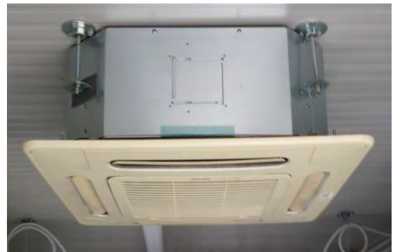
Figure 22. Air conditioner system installed in the greenhouse
