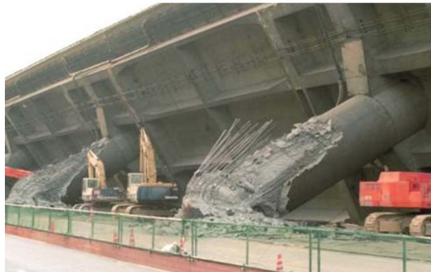
Figure 1.22. Insufficient number of stirrups for shear (Hanshin expressway, Kobe, 1995)
