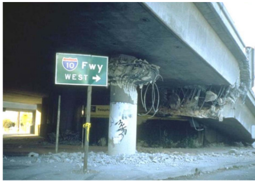
Figure 1.21. Insufficient confinement of columns (Northridge, California 1994)
