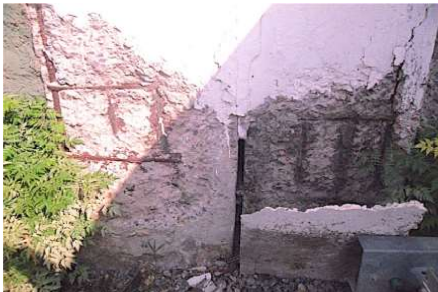
Flexural cracks in RC beams (Haseeb Jamal, 2018)
