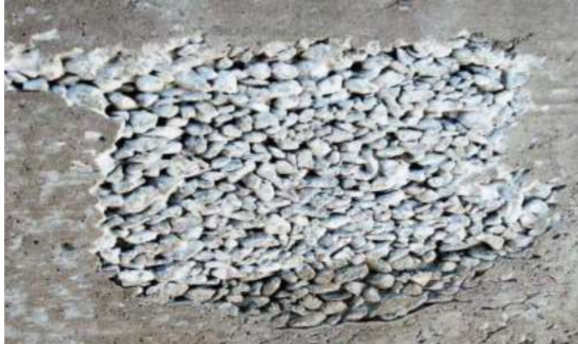
Honey combing in concrete (Haseeb Jamal, 2018)
