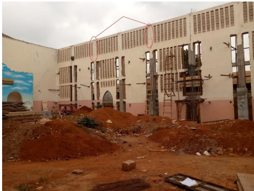
Figure 3.3. The state of the building during the site visit showing cracks (onsite picture, 2022)
