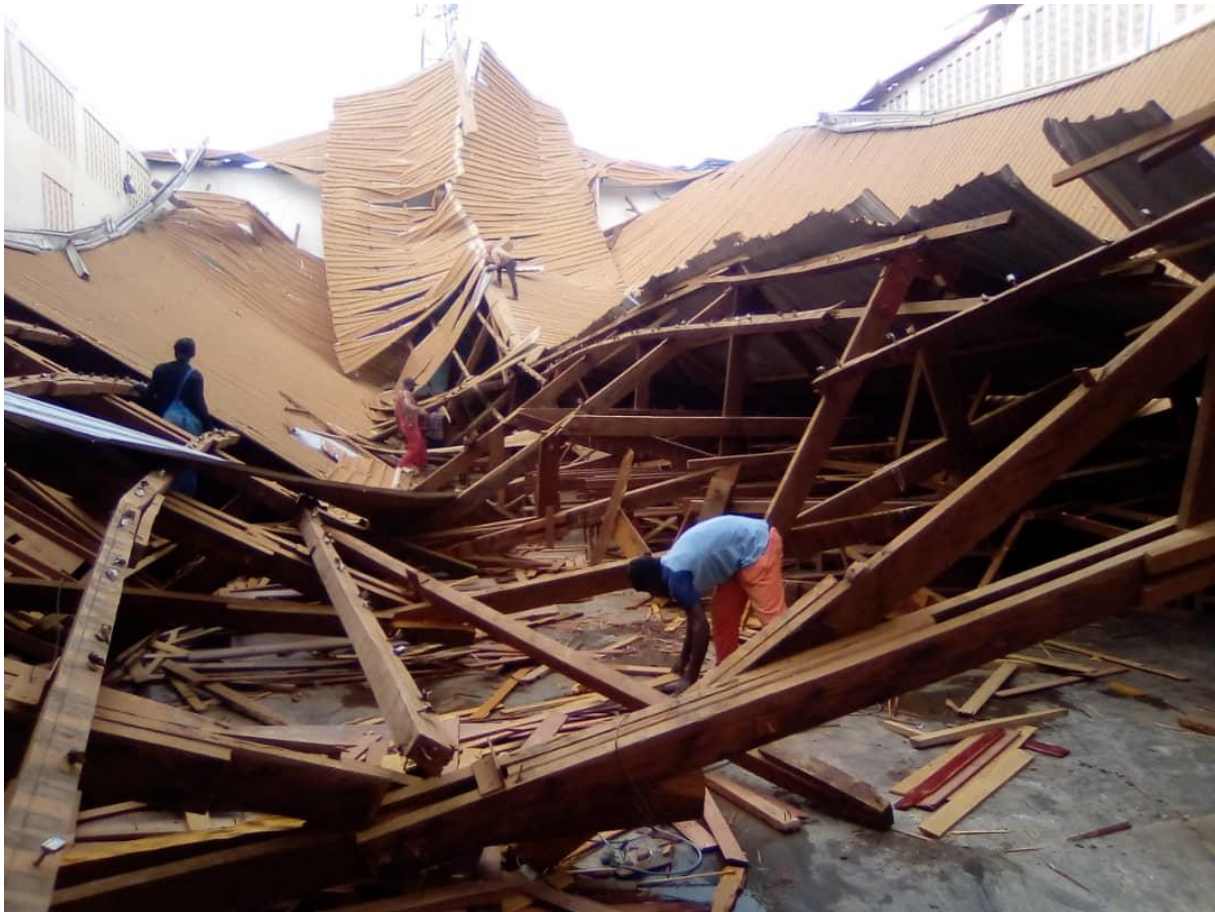
Figure A.5. The collapse of the roof of EFLC Mimboman (03/08/2020, 9:45 am)
