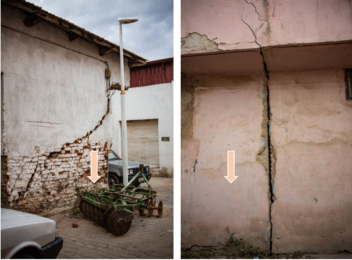
Figure 2.8. Damage to buildings in the Sarıgöl district caused by earth fissure (photos by Can Yüksel, 2023).
