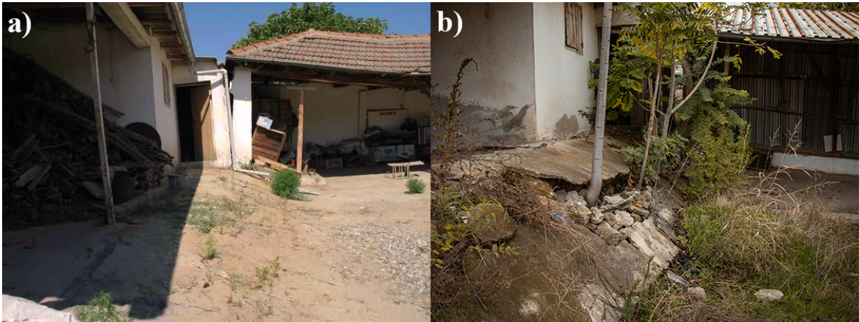
Figure 6.2. Comparison photos of land subsidence in the Sarıgöl district for same location (for photo locations, see Figure 2.3-6). a) Photographed by Demirtaş (2008). b) Photographed by Yüksel (2024).
