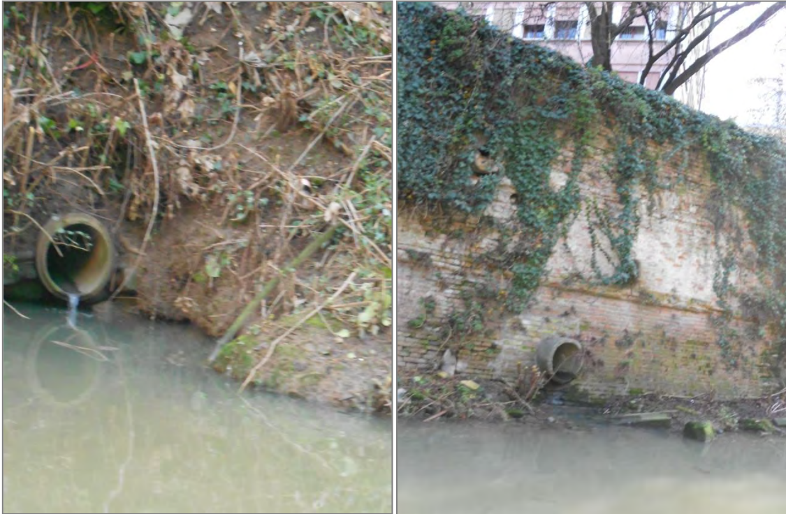
Figure 2-12 Sewage release in Piovego channel.
