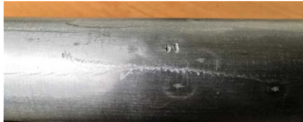
Figure 7.8: Worst damage point in the HV electrode.
