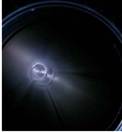
Figure 4.23: Picture of installed electropolished pipes with mirror-like surface.
