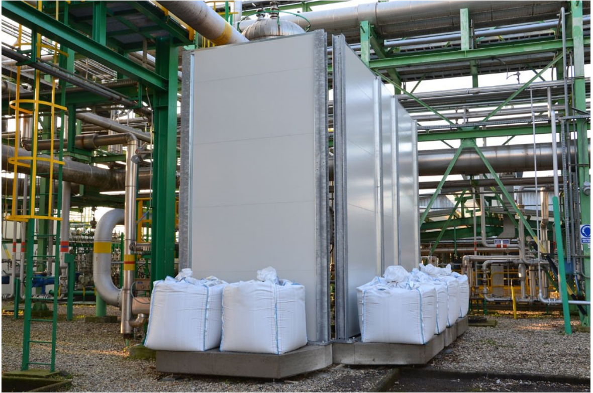
Figura 4.7 – Barriera antirumore mobile
