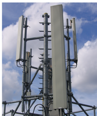
(a) Base Station GSM/GPRS.
