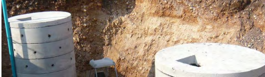
Figure 1.8. Infiltration well for artificial recharge situated at Cornedo Vicentino (Vi) [57]
