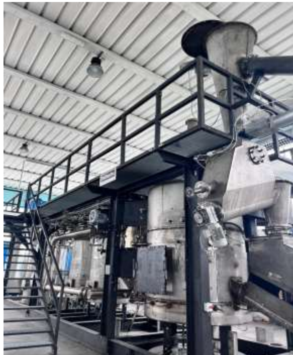
Figure 2. 4: Overview of the pyrogasification plant
