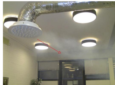
Figure 11 Supply air terminal device and airflow evidence provided by smoke machine.
