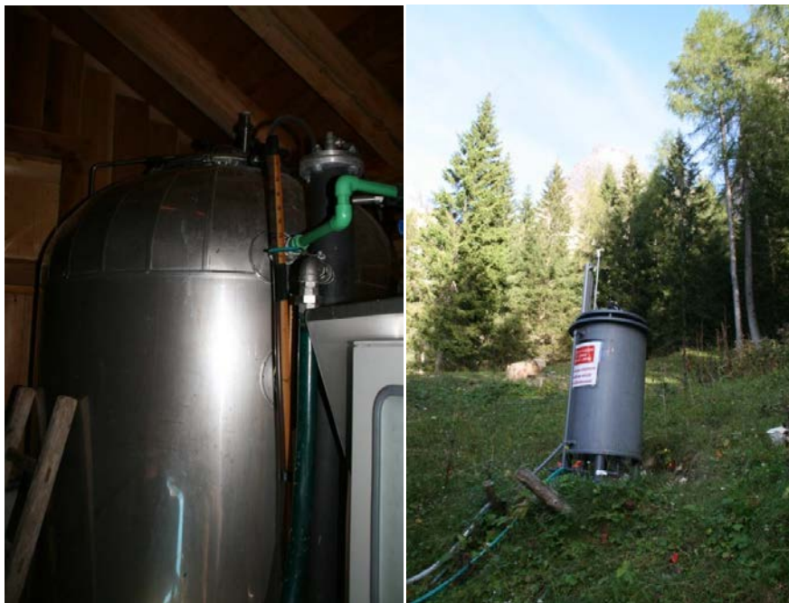
Figure 2.3 Anaerobic digester (left) and gas bell (right) installed at Bosconero hut.
