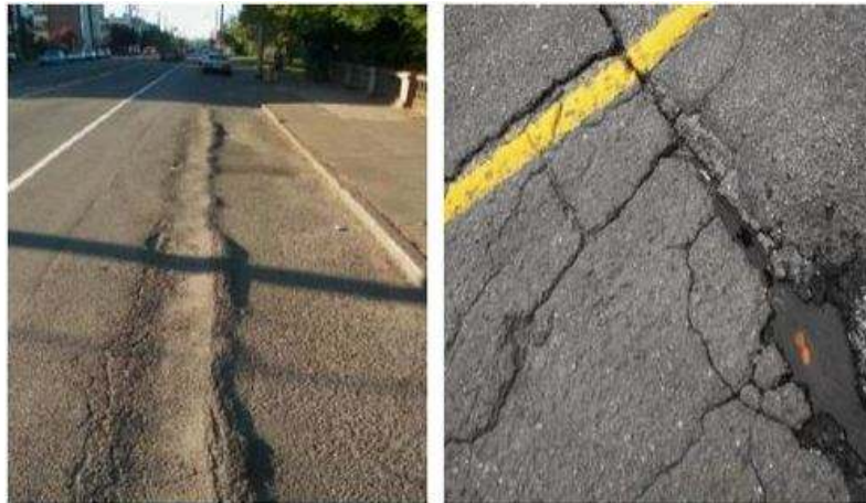
Figure 1.8. Pavement Rutting ( http://www.sptc.org/briefs/2016/5/17/evaluating-ruttingstripping-potentials-of-asphalt-mixes-using-hamburg-wheel-tracking-device )
