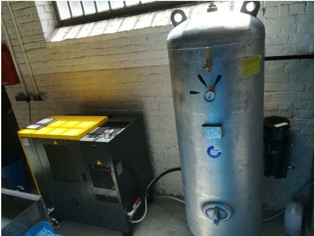
Figure 8: External compressor and storage tank
