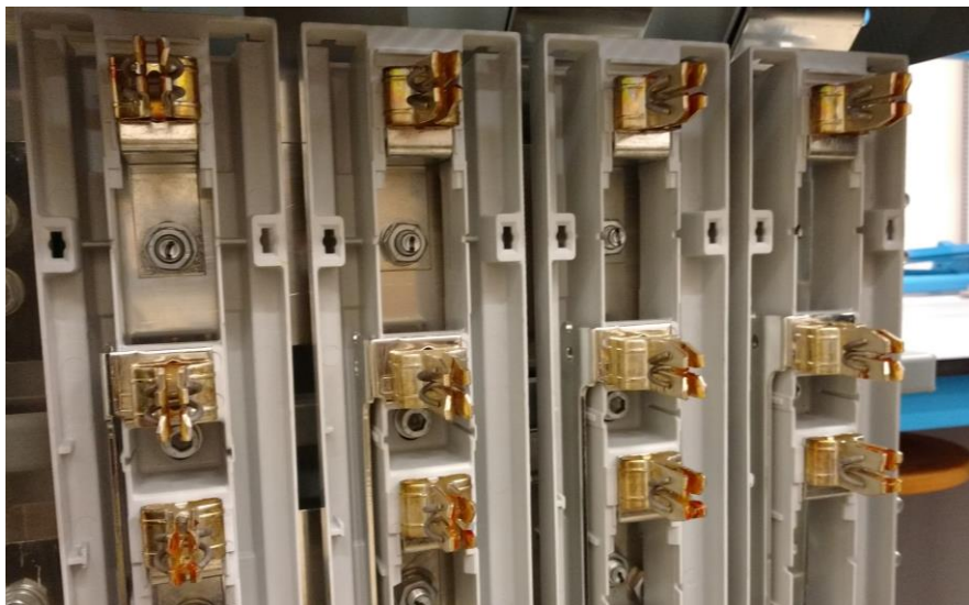
Fig. 3.4 Holders for the fuses.
