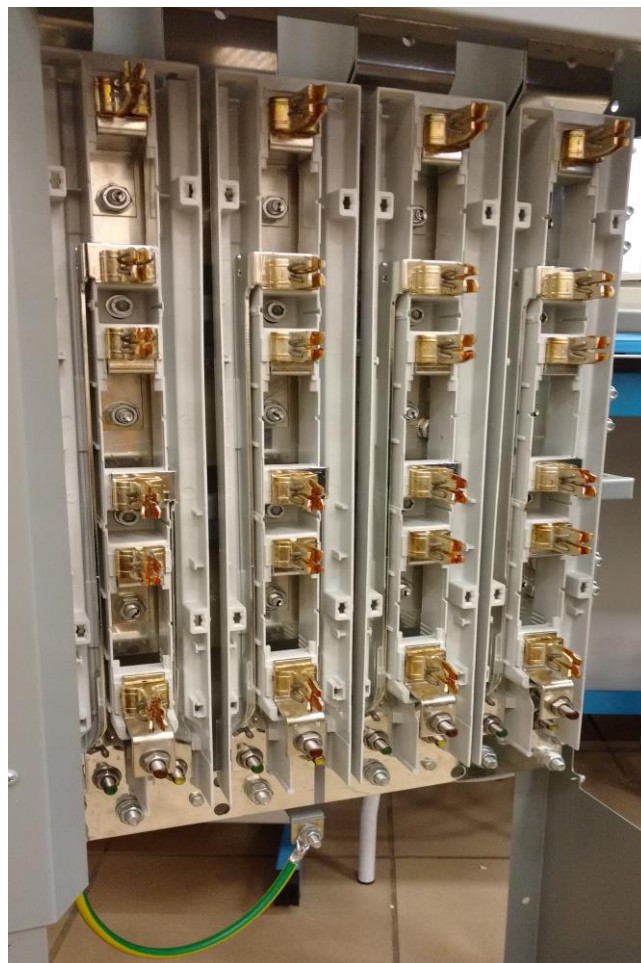
Fig. 3.1 Photo of the electrical distribution panel.
