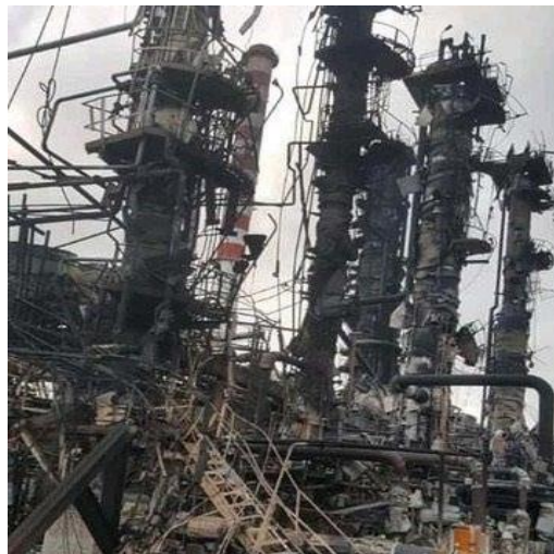
Figure 1.23. Damaged SONARA structure ( https://thesuncameroon.cm/huge-explosion-fire-ravage-sonara )
