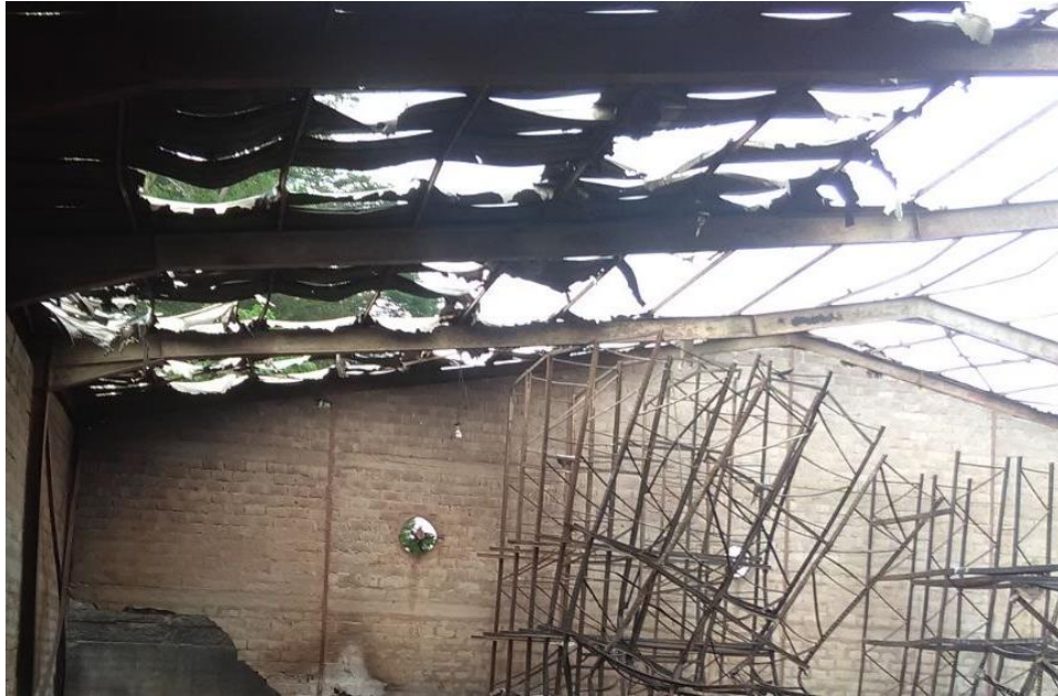
Figure 3.10. Damaged roofing elements due to fire
