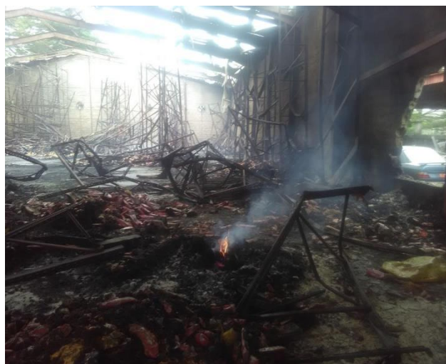
Figure 3.2. Panzani's warehouse directly after fire damage
