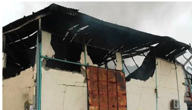
Figure 1.25. Damaged structure of Biopharma's warehouse ( https://www.cameroon-tribune.cm/article.html/21978/fr.html/incendie-biopharma )
