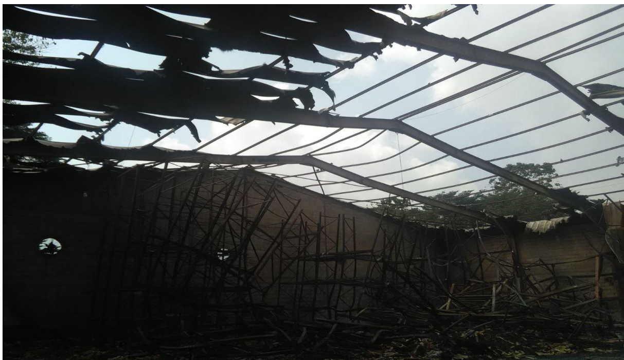
Figure 3.13. Damaged roof elements of the Panzani's store
