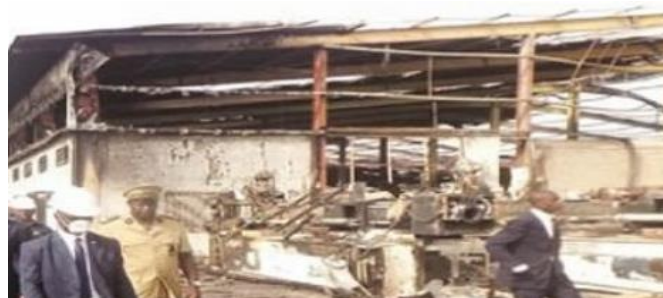
Figure 1.24. Damaged structure of FERMENCAM warehouses ( https://www.cameroun24.net/blog/?pg=actu&ppg=1&pp=&id=4359 )
