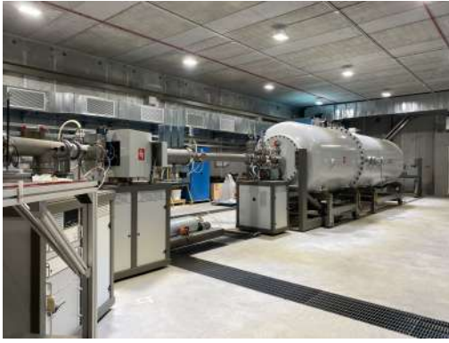
(a) Accelerator installed at LUNA MV.
